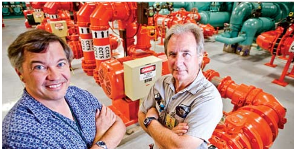
PHOTO: Site Services engineer Art Kienle (left) and mechanic Doug Macpherson helped replicate water and cost savings from Kent, Wash., to El Segundo, Calif. GLADYS WICKERING/BOEING
