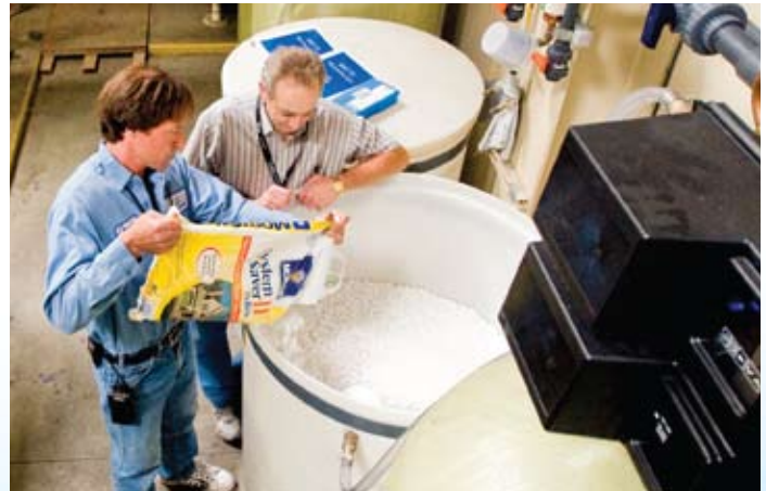
PHOTO: Boeing heating, ventilation and air-conditioning mechanic Brett Weberg adds salt used in regeneration tank for cooling-tower water softeners at the Kent, Wash., site. The water softener is part of a new process initiated by lead mechanical engineer Roger Sampair (right) that will save water and reduce sewage and maintenance costs across Boeing. MARIAN LOCKHART/BOEING
