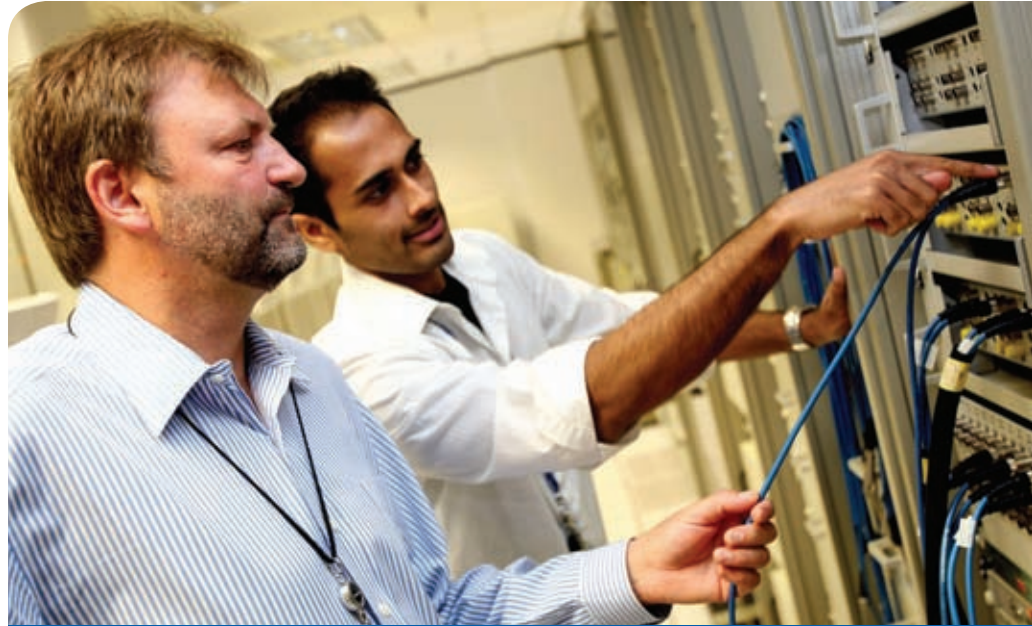
Manfred Hornung (left), manager of the Boeing International Space Station Software Development and Integration Laboratory (SDIL) Support Systems, and Neel Sheth, software engineer, are inspecting bus connections in the SDIL computer room. Boeing recently won a NASA award for improving the way the SDIL is used. PATRICK ARMSTRONG PHOTO
