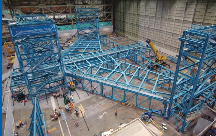
Construction is under way on the superstructure that will be used to static test the Boeing 787 Dreamliner. The steel structure is 208 feet (63.4 meters) wide, which allows a free span greater than the wingspan of the 787 airframe.
