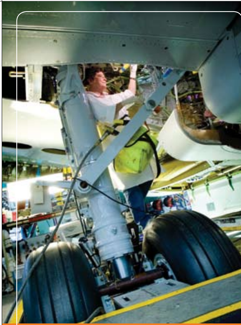
Sealer Barbara Rogers applies anticorrosion sealant to the 737 wheel well. 737 engineers have adapted a technique used on the F/A-18 to make installation of the wheel-well hydraulics more efficient.
